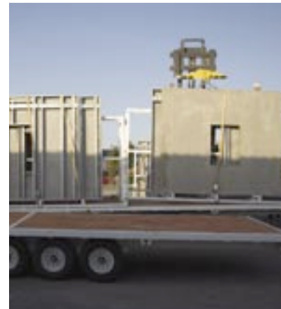
Walls are stacked onto special A-frames for loading onto light-duty trailers for early-morning transport 45 miles to the job site. In spite of 10 miles of rough, wash-boarded dirt road, the panels arrived intact.
